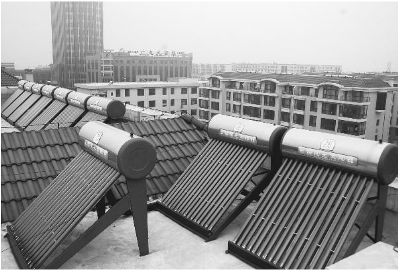
Solar evacuated tubes heat the water on a roof in Rizhao, China.
